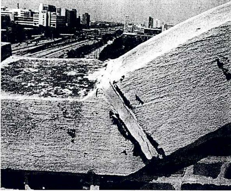
Figure 15. Failure of the sealant at joints in the limestone coping.
