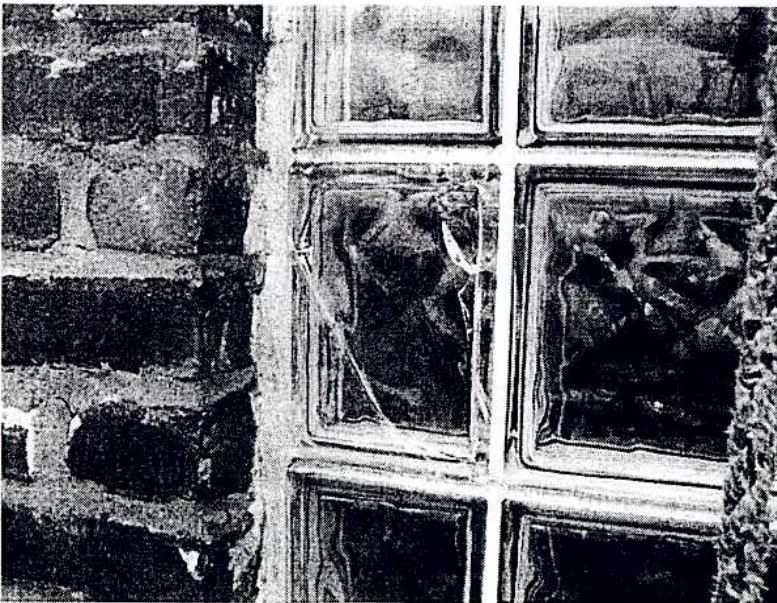
Figure 20. Cracked glass block along west elevation.
